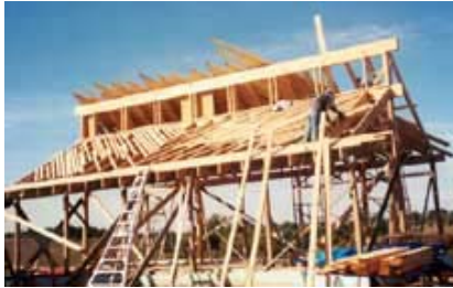
Fig 12: Test house under construction, all framing from locally harvested and milled lumber
